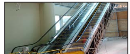
New north elevators from ticketing to mezzanine will open later this summer.
